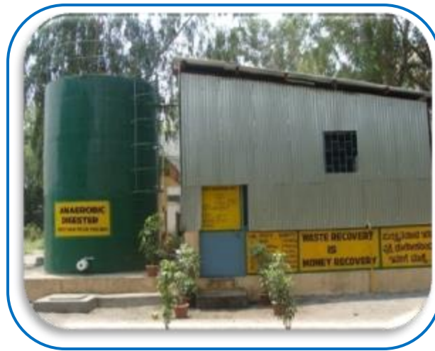
Bio gas plant at colony
