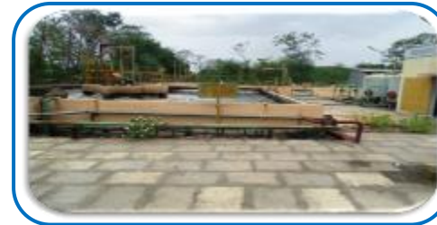
New clarifier - STP
